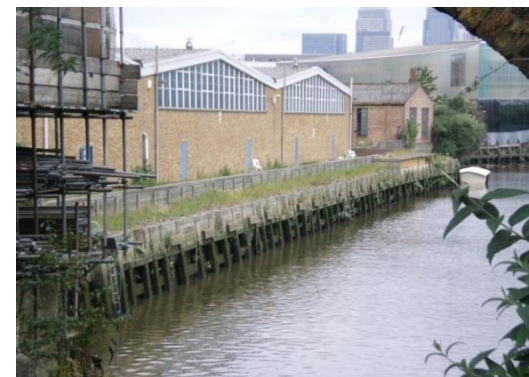
AFTER – This flood defence wall was set back to create a vegetated terrace, and a sandbank for birds ©Environment Agency
