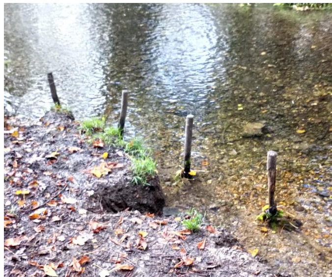
Figure 16, Evidence of bank erosion in Reach 3.
