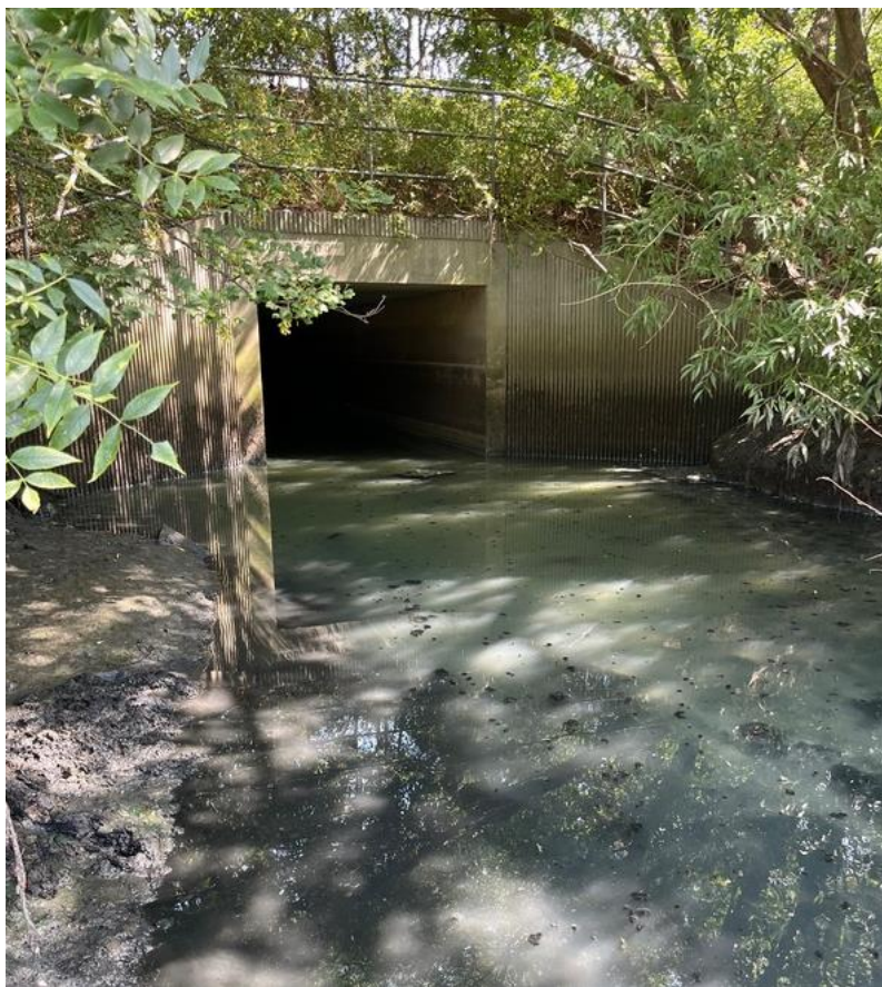
Figure 11: One of the only open air sections of the Cranbrook, close to the confluence showing visual evidence of pollution
