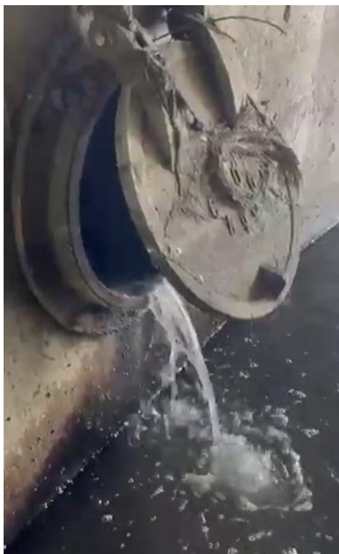
Figure 29: Still from a video of discharge from the outfall at Ilford Hill Bridge.
