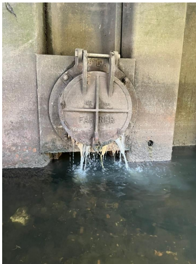
Figure 21: outfall at Aldersbrook showing evidence of sewage pollution
