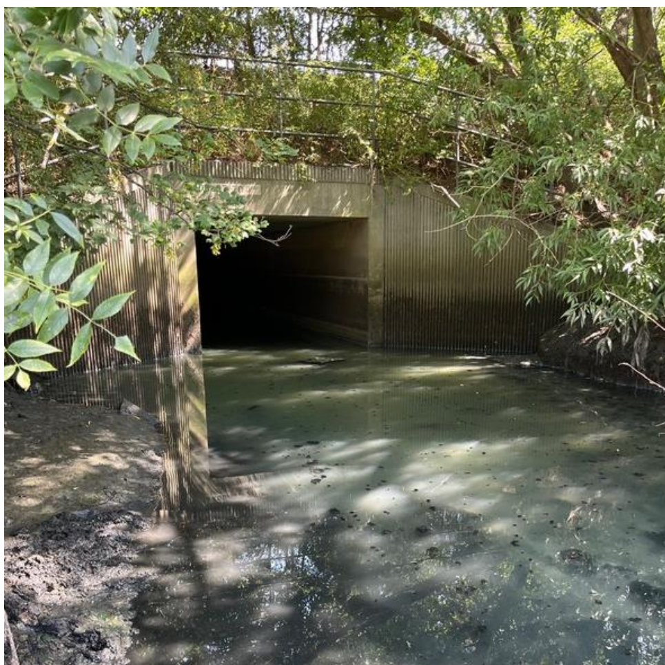
Figure 1: One of the only open air sections of the Cranbrook, close to the confluence showing visual evidence of pollution
